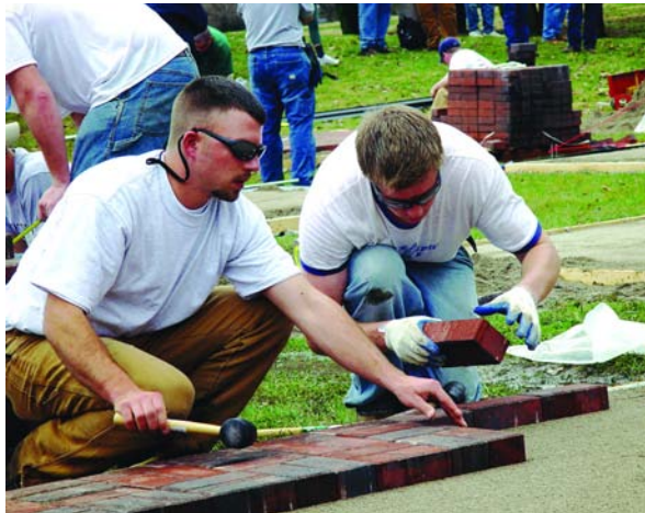
Students Mark Maslow and Nick Dangl work together in the patio construction event.
